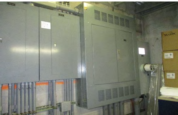
29 Breaker Panel Overview
