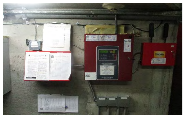
32 Security Alarm Overview
