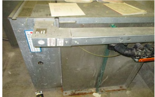
36 Elevator Motor Overview
