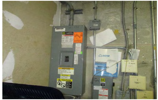
34 Breaker Panel Overview
