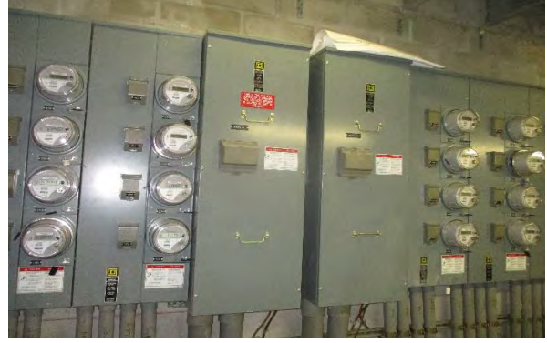
28 Breaker Panel Overview
