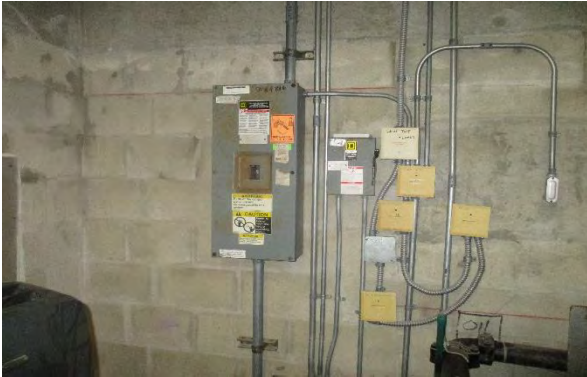
43 Breaker Panel Overview
