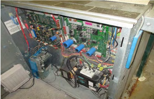
35 Elevator Control Board Overview
