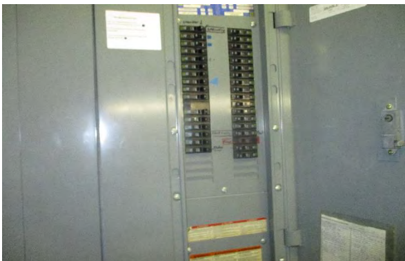
31 Breaker Panel Overview
