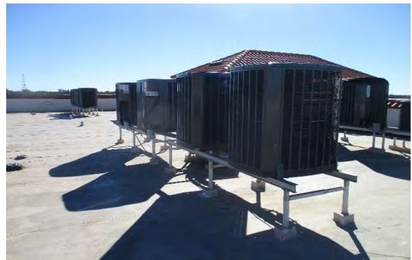
38 HVAC Stand/s Overview
