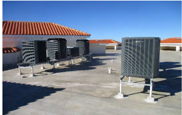
44 HVAC Stand/s Overview
