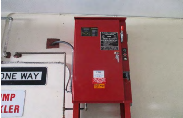
27 Fire Alarm Overview
