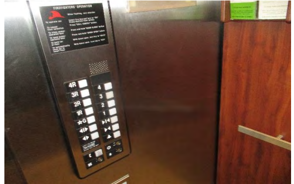
60 Elevator Control Overview
